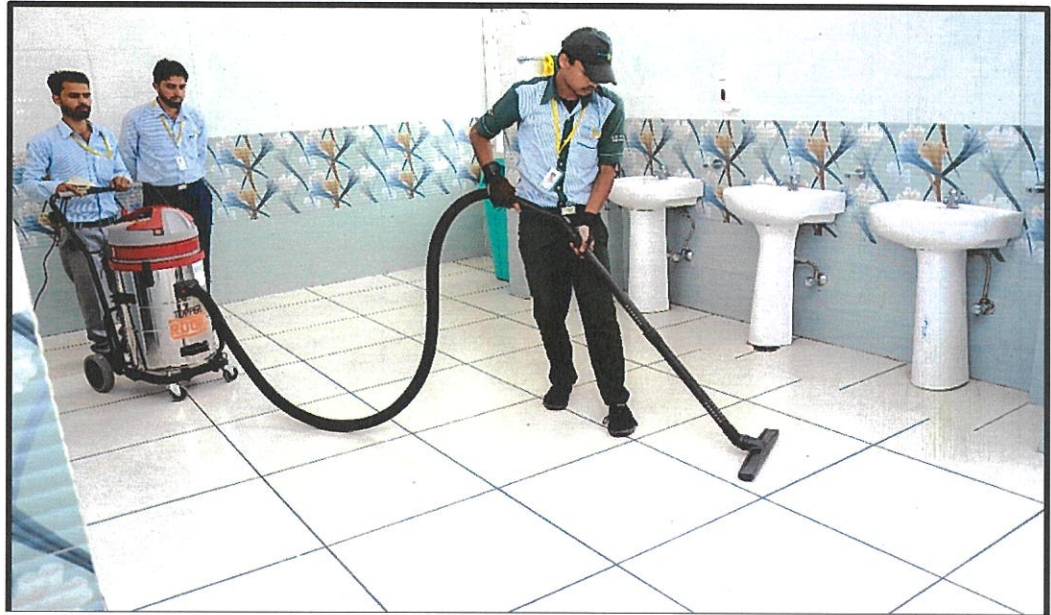
Vacuum cleaners and water pressure jet machines being used on Tarakote Marg for cleaning of toilets
